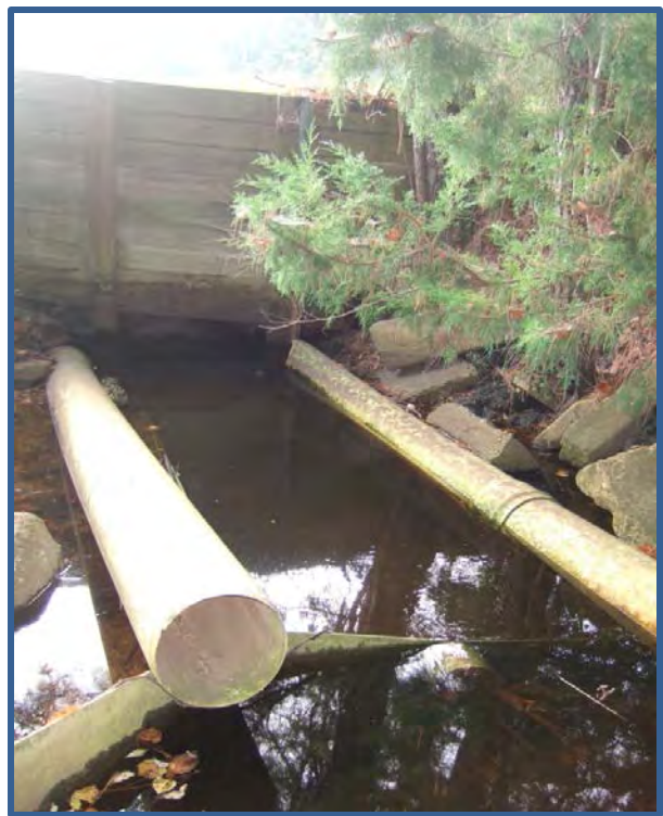
Figure H-1 A wide variety of stormwater management concepts have been tried in the past. This is the remnants of a chlorine contact chamber designed to treat water draining upstream of the Bike Bridge in Georgetown County. (Photo courtesy of Dr. Dan Hitchcock, Clemson University)
