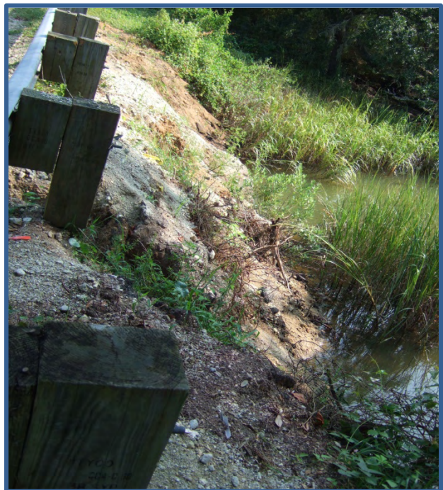
Figure H-9 Example of a poorly stabilized roadway construction project resulting in significant erosion directly into one of Murrells Inlet's tidal creeks. (Photo courtesy of Dr. Dan Hitchcock, Clemson University)
