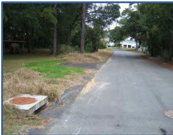
Figure C-9 Conventional storm drain which directs runoff untreated into the nearest waterbody (Photo courtesy of Dr. Dan Hitchcock, Clemson University)
