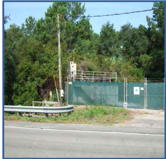
Figure G-1 Georgetown County WSD force main pump station equipped with the SCADA monitoring system. (Photo courtesy of Dr. Dan Hitchcock, Clemson University)
