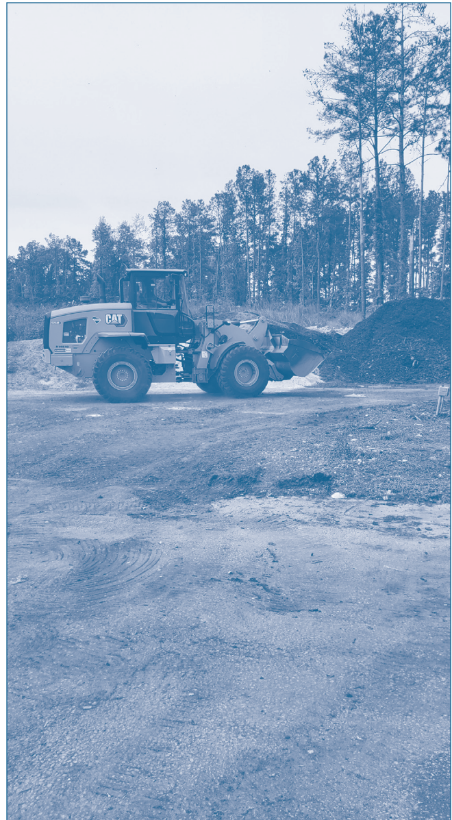
Pictured is a tractor working a windrow at a Midlands composting facility.
